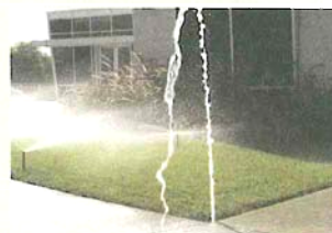
Geyser due to missing nozzle or broken sprinkler
